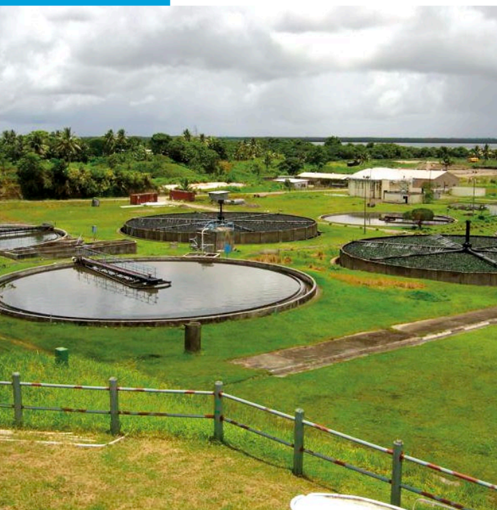
Kinoya Sewerage Treatment Plant in Fiji where Biogas Capture and Flaring is being implemented
